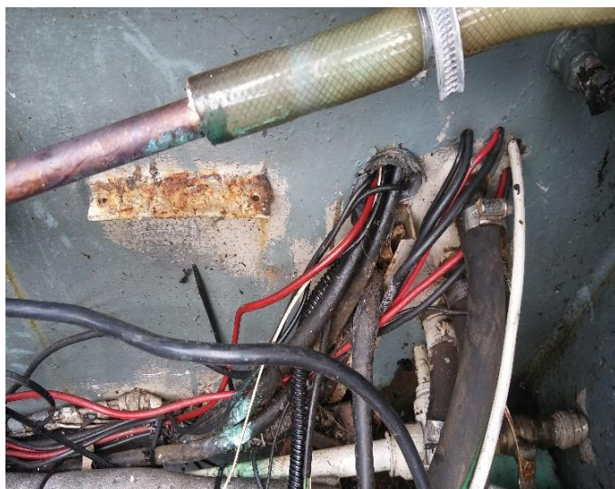
Figure 16 Poor cable routing and support
