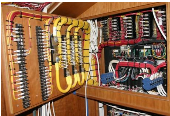
Figure 2 DC switch/panel-board wiring
