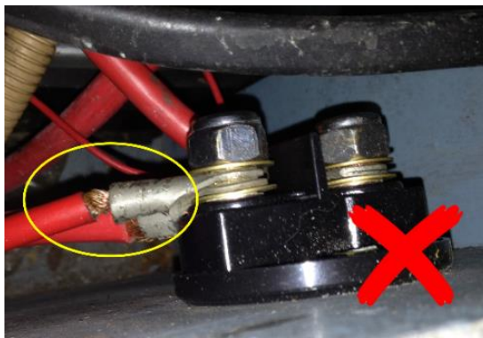
Figure 5 Non-compliant exposed terminal lug shank on a +12 V connection to a battery isolation switch
