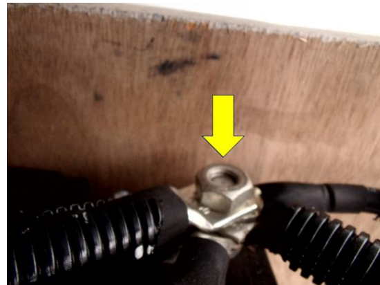
Figure 15 Inadequate battery cable retention
