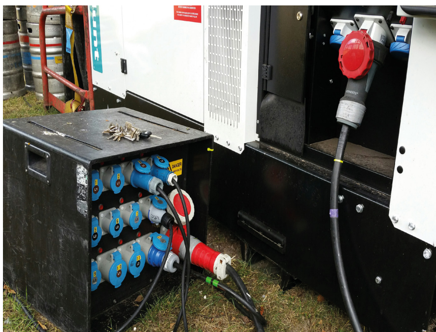
Figure 1 Distribution board fitted with plug and socket connectors
