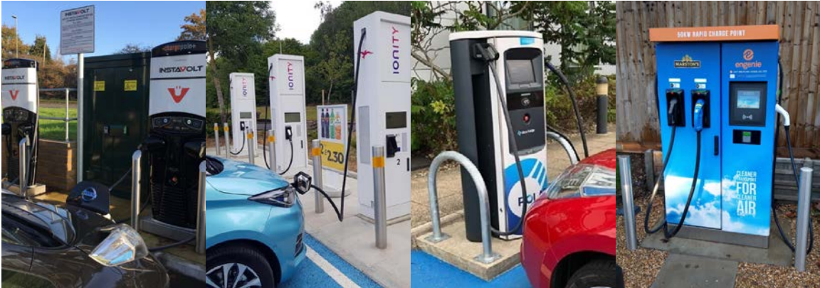
Figure 4.4 Example rapid and ultra-rapid chargepoints
