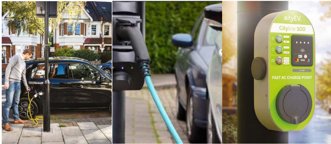
Figure 4.6 EV charging integrated with street lighting: Ubitricity, Char.gy and City EV. Reproduced by permission of Ubitricity and City EV
