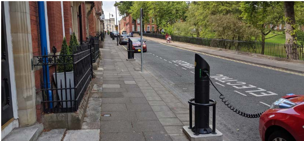
Figure 4.10 On-street residential long-stay charging
