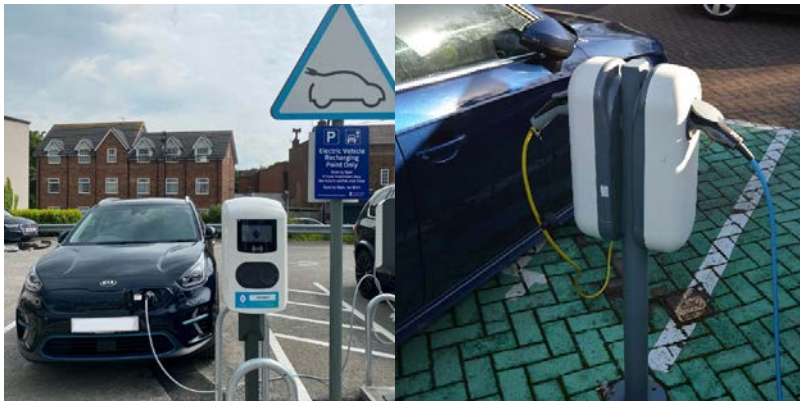
Figure 4.2 Example post/pedestal-mounted chargepoints
