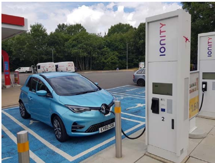
Figure 4.13 Ionity ultra-rapid chargepoints at a motorway service station
