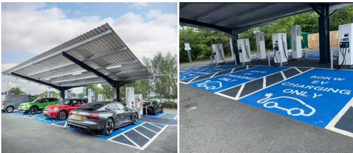
Figure 4.12 EV charging hub in Stretford, Manchester
