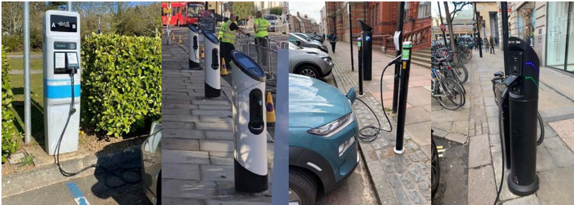
Figure 4.3 Example free-standing AC chargepoints
