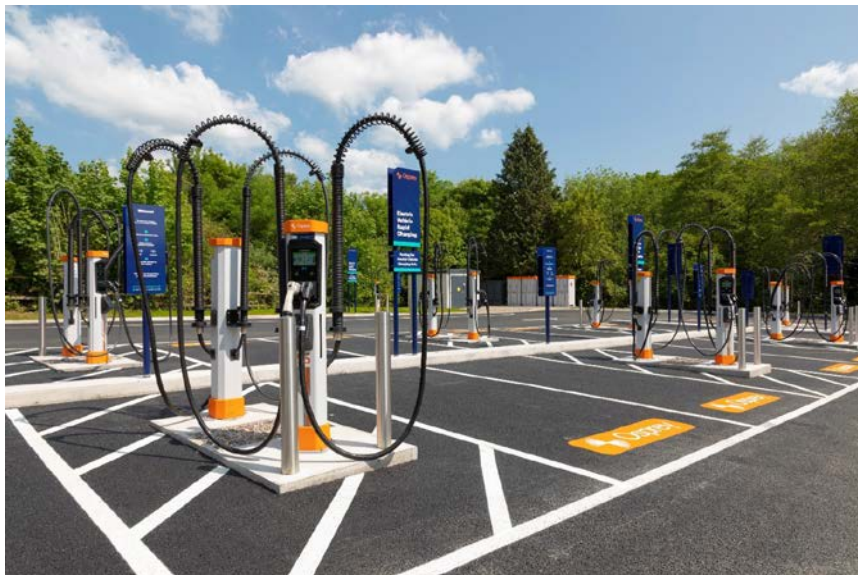
Figure 7.6 Osprey's 16 high-power chargepoints at Salmon's Leap are compatible with every rapid-charging vehicle on the market. Reproduced by permission of Osprey Charging Network
