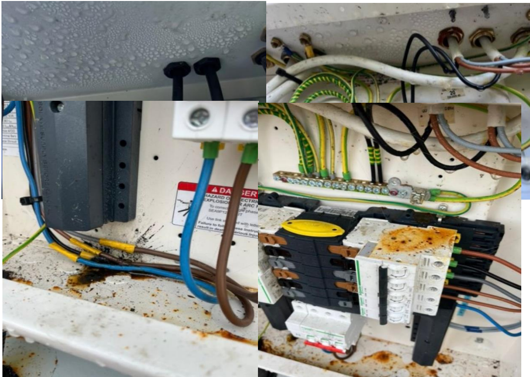
Figure 4 More extreme examples of condensation in an enclosure that had protection by an additional GRP enclosure but no additional measures in place. The condensation here caused a fault (bottom right)
