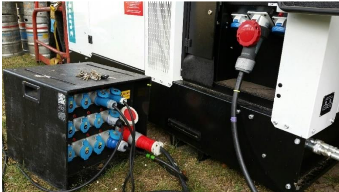
Figure 1 Distribution board fitted with plug and socket connectors
