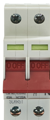
Figure 2 Main switch disconnector (Reproduced with permission of Electrium)
