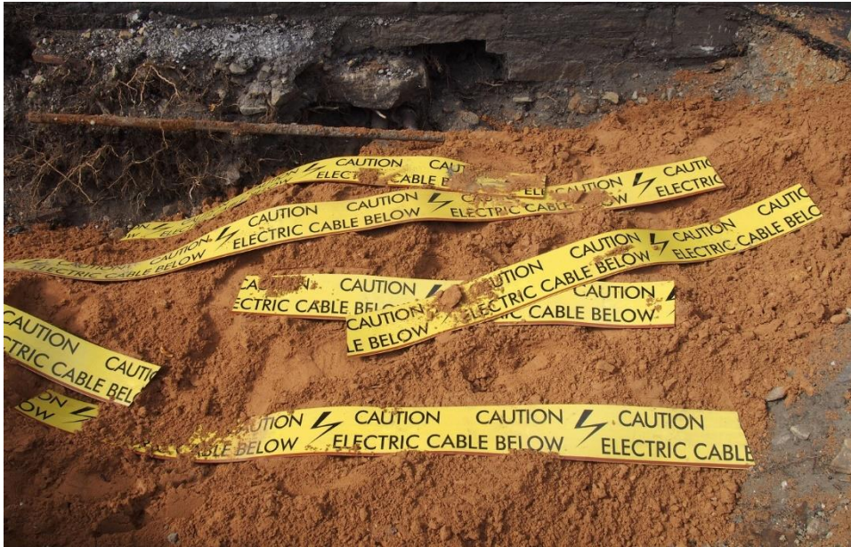
Figure 1 Cable marker tape
