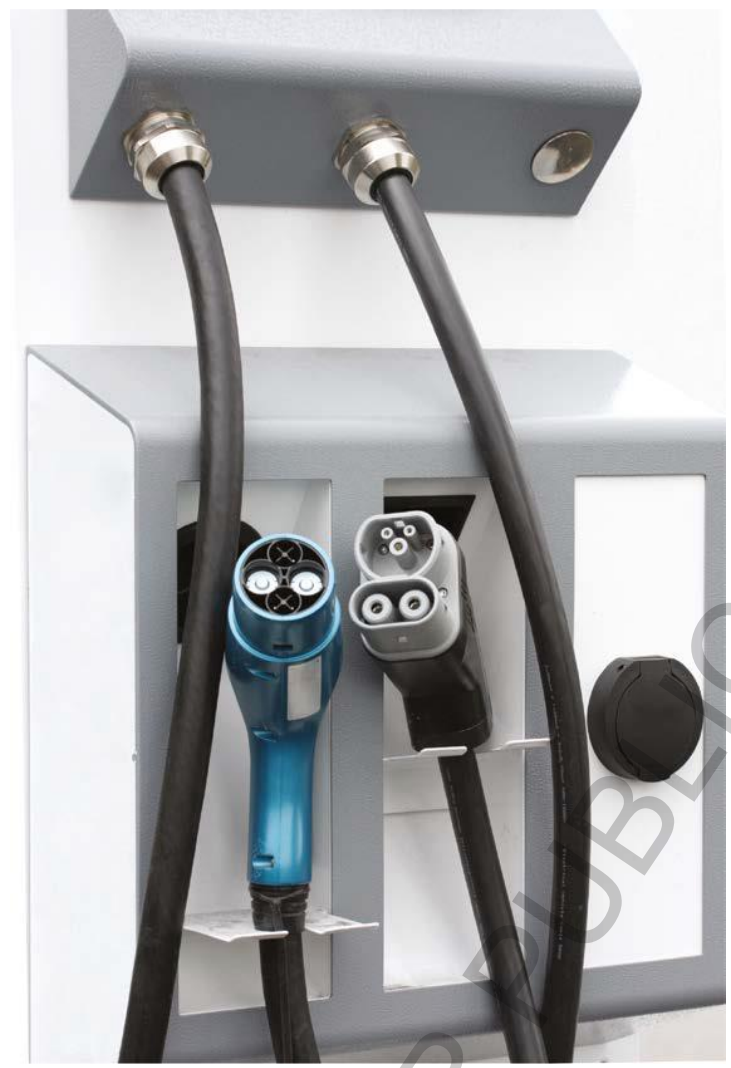
Figure A.6.A.4 Mode 4 Charging – charger with both combined charging system (CCS) and CHAdeMo tethered outlets
