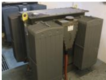
Oil-filled substation transformer
