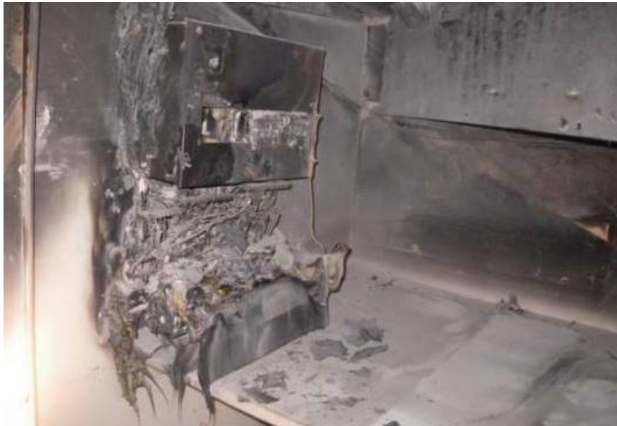
This photo shows a fire involving a plastic consumer unit (bottom) and a metal consumer unit (top). In the experience of the LFB, when a fire originates within a metal consumer unit (even without sealed grommet holes and the plastic MCB cover failing), the fire is still generally contained to the consumer unit.
