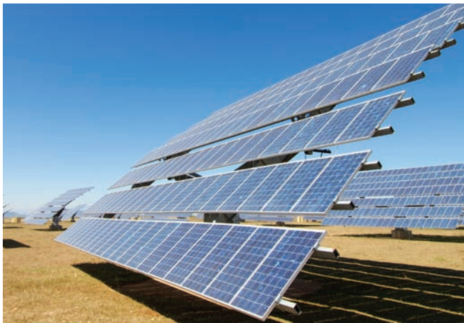
PV system on open ground
