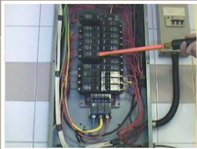
Fig 7: Positive image of an MCB in a distribution board
