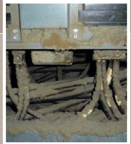
Fig 4: Accumulation of dust in equipment
